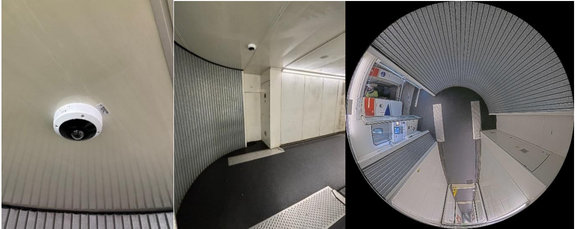
Figure 1: Example Internal Passenger Boarding Bridge camera installation & view
